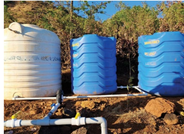
Water Tank for Watering
