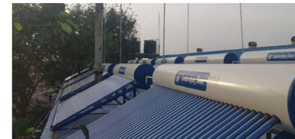
Devlapar Solar Water Heater
