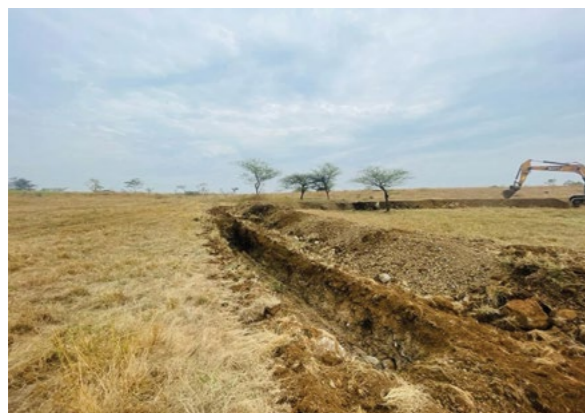
Water Absorption Trench
