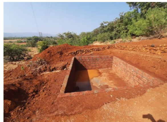
Water Storage Tank for Watering
